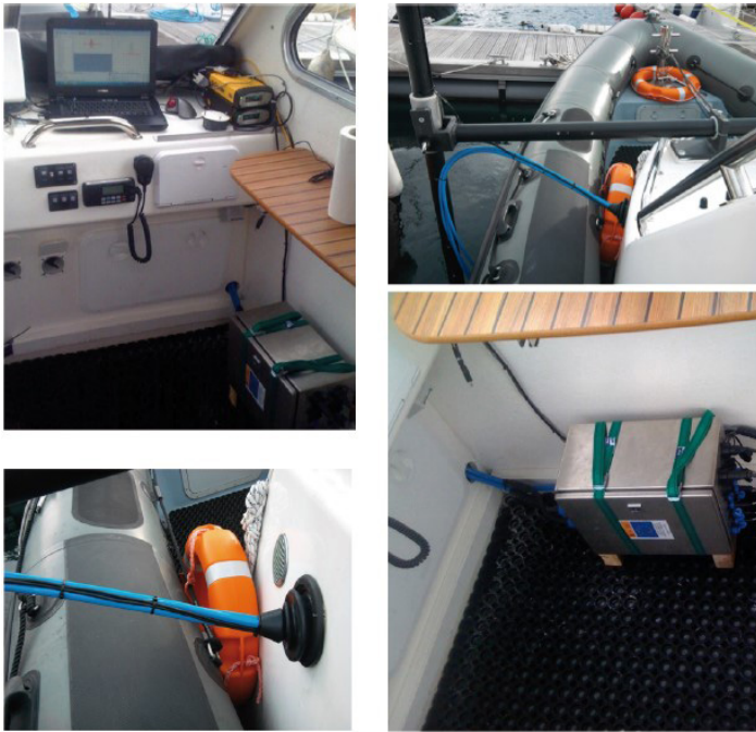
Fig. 3. Detail of the installation of the operating unit within the cabin under the folding table and the top right are seen the GPS in yellow. The solution adopted is also shown for output cables to the transceiver unit in the two photographs bottom of the figure.
