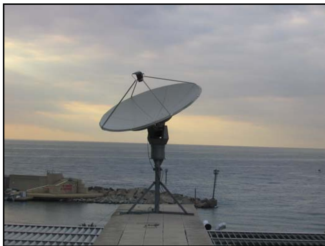
Fig. 2. HRPT old receiving system
