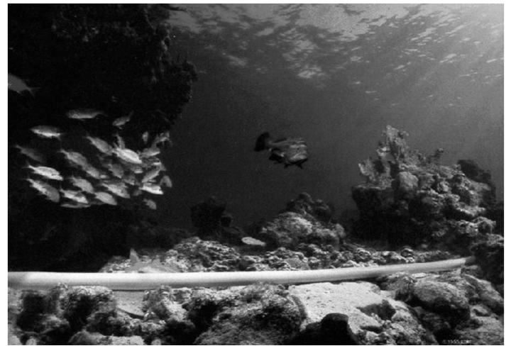
Figure 2. Submarine cable on seabed
